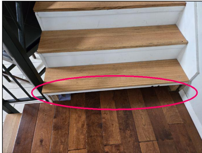
Missing rising on main staircase.
