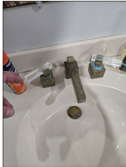
Faucet corroding in master bathroom sinks.
