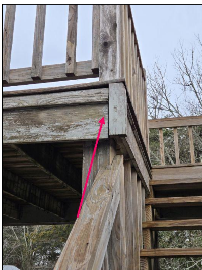
Joists starting to pull away from each other.
