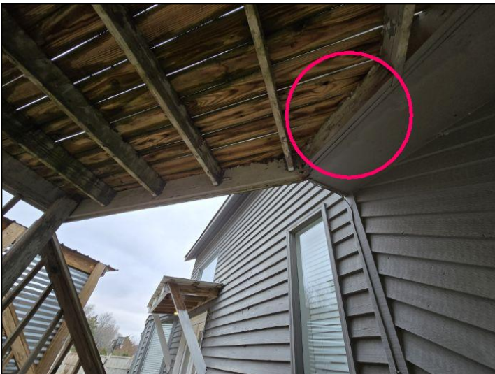
Deck not properly mounted to home.
