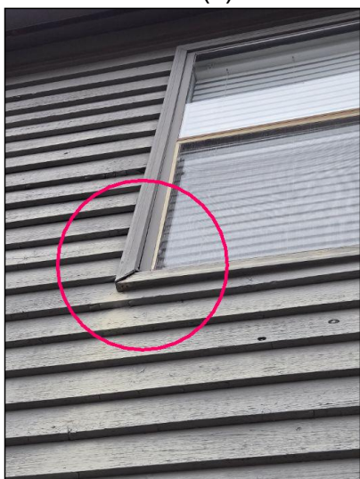
Deteriorated frame(s) at window(s)
