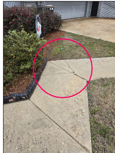
Small cracks in walkway. Should be monitored.
