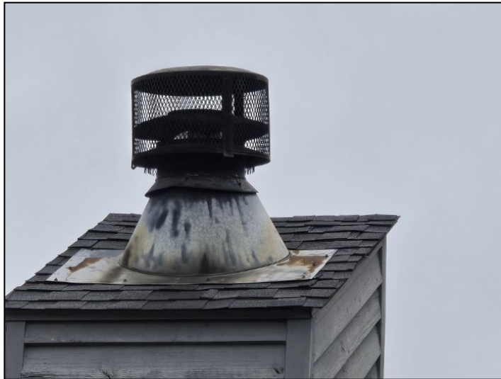
Chimney cap not properly sealed or covered.
