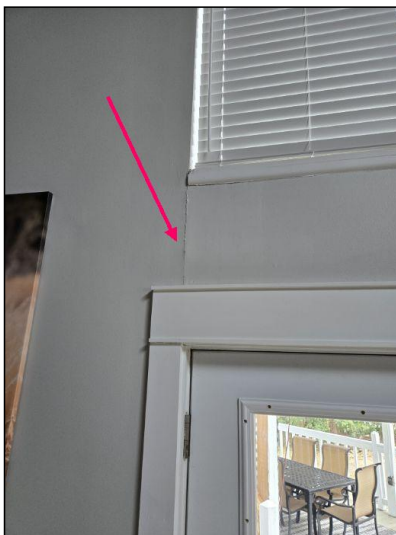
Settlement cracking. Should have a professional look at and repair.
