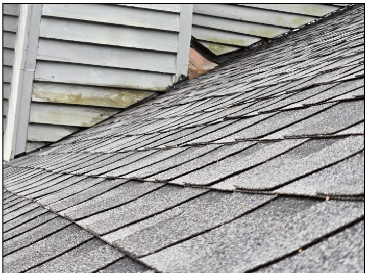
Recommend review by a licensed roofer for repair or replacement as necessary.
