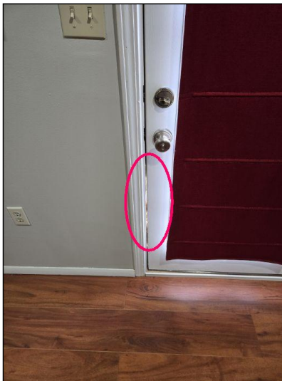
Doors do not seal well. this can be an energy drain.
