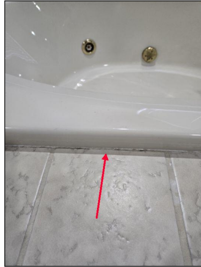
Caulking needs to be redone
