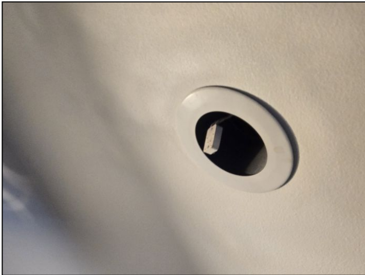
Light bulbs missing in dinning room.
