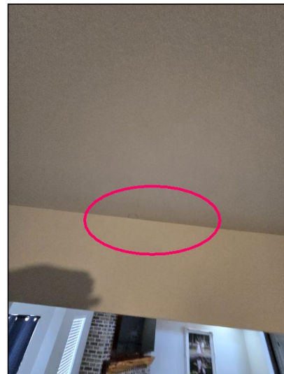
Possible water damage.
