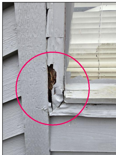
Deteriorated frame(s) at window(s)
