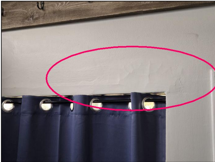
Paint bubble due to possible water intrusion.
