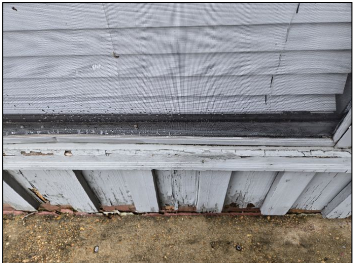
Deteriorated frame(s) at window(s)
