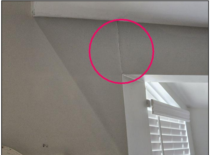
Small cracking. Possibly from settlement of house.
