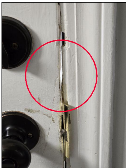
All exterior doors needs the seals replaced.
