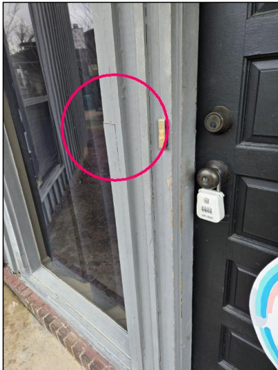
Frame separating from glass
