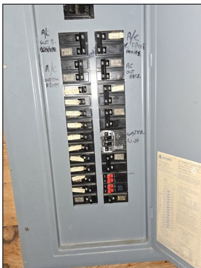
Electrical panel not properly labeled.
