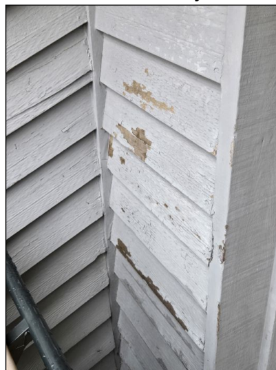
Some areas need priming and repainting.
