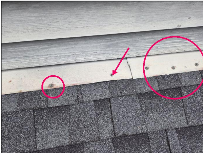
Missing screws in flashing, and screw heads should be sealed to prevent water damage.
