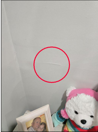
Paint bubble in left rear bedroom. Possibly from water.
