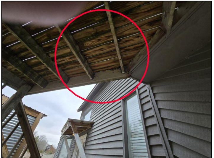
Severe water damage to decking. Should have a professional check before use.
