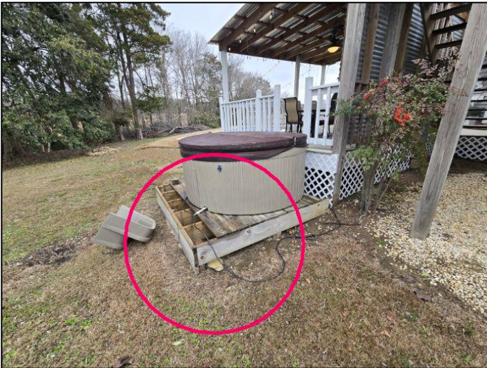
Hot tub decking falling apart, and has water damage.
