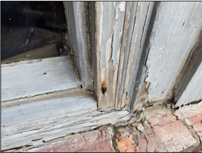
Deteriorated frame(s) at window(s)
