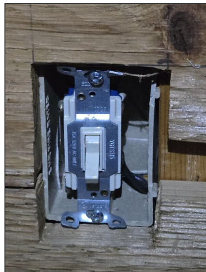
Cover plate missing.
