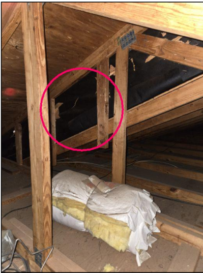
Wall paper torn in several spots. Can see daylight through wall.
