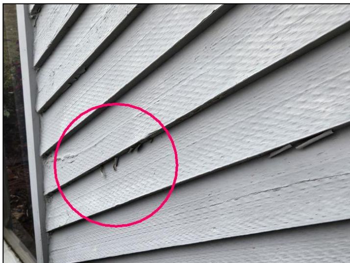
Some areas need priming and repainting.
