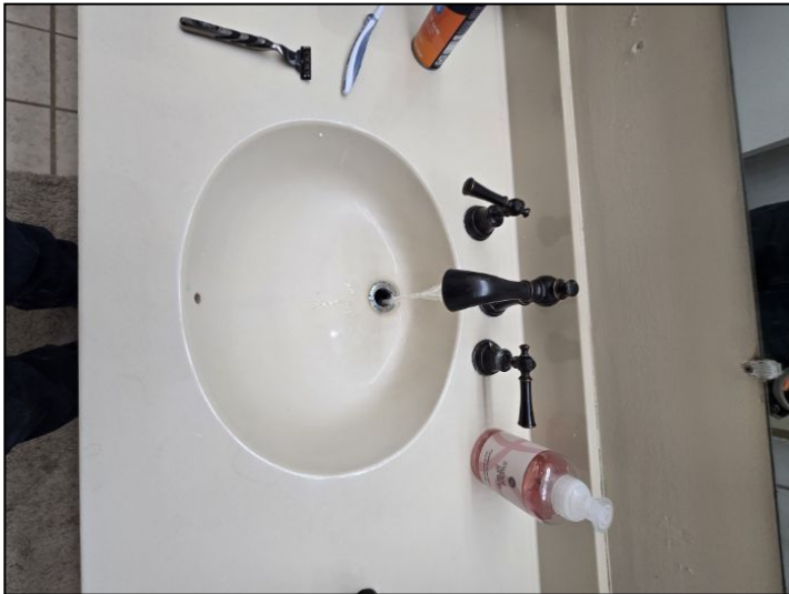
No stop in sink. Hot water not working.
