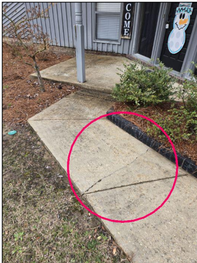
Small cracks in walkway. Should be monitored.
