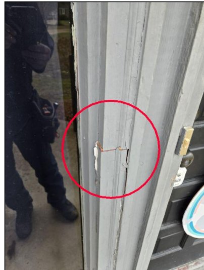
Frame separating from glass
