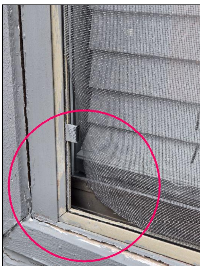
Some window screens damaged.
