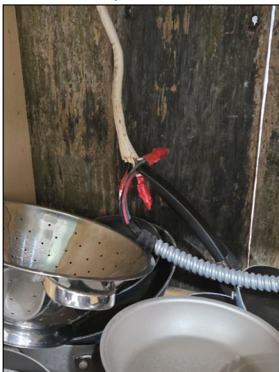
All electrical connections should be located in a junction box.
