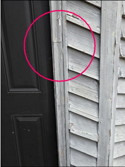
Wood deterioration observed. Suggest repairs/replacement as needed.
