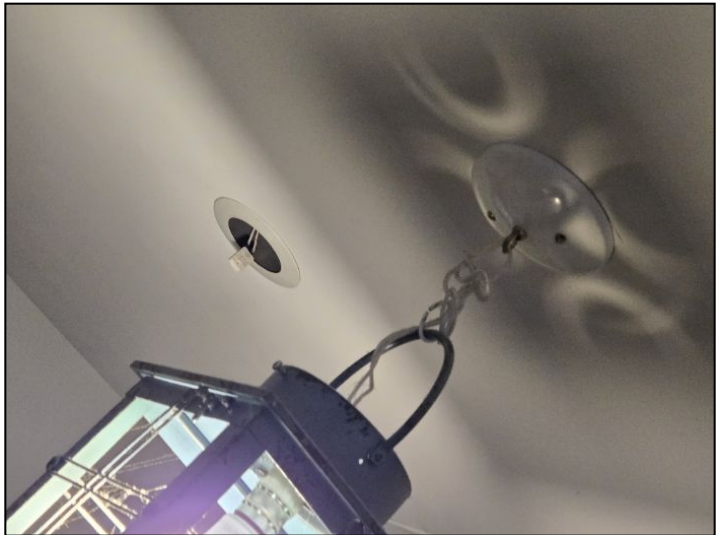
Light bulbs missing in dinning room.
