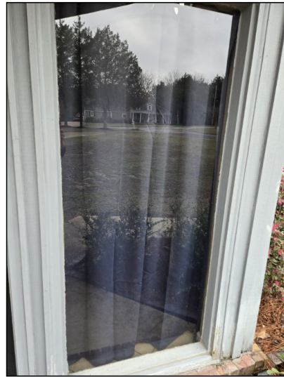
Suggest caulking around doors and windows as necessary.
