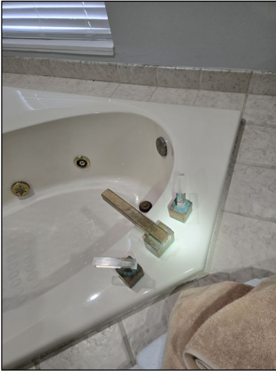
Hot water did not warm up. Fixtures are starting to corrode.
