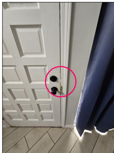
All exterior doors needs the seals replaced.
