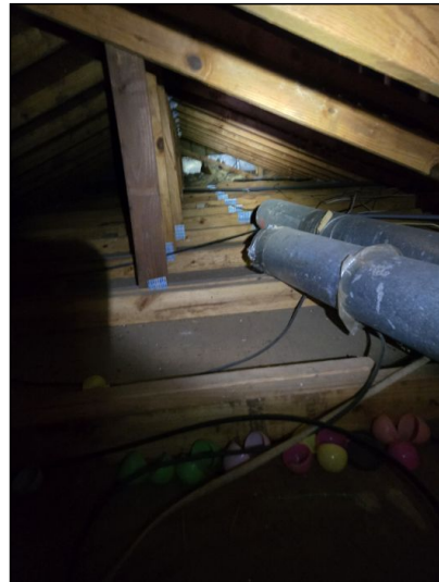
Insulation is sparse in some areas.
