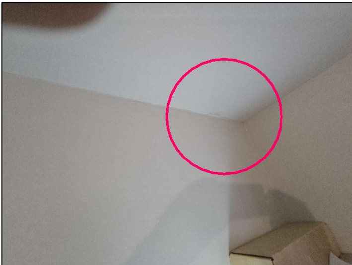
Possible water damage.
