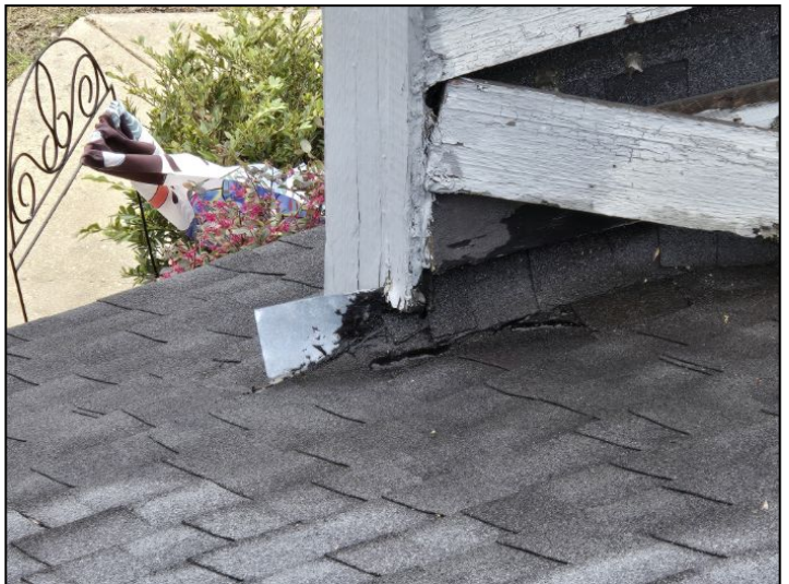
Some wood deterioration noted. Have repaired as necessary.
