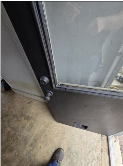
Wood deterioration observed. Suggest repairs/replacement as needed.
