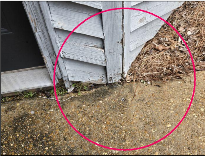
Siding in contact with ground.
