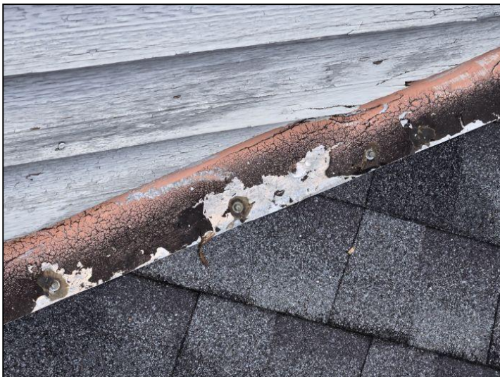
In the inspectors opinion the flashings are near the end of their useful life due to wear.
