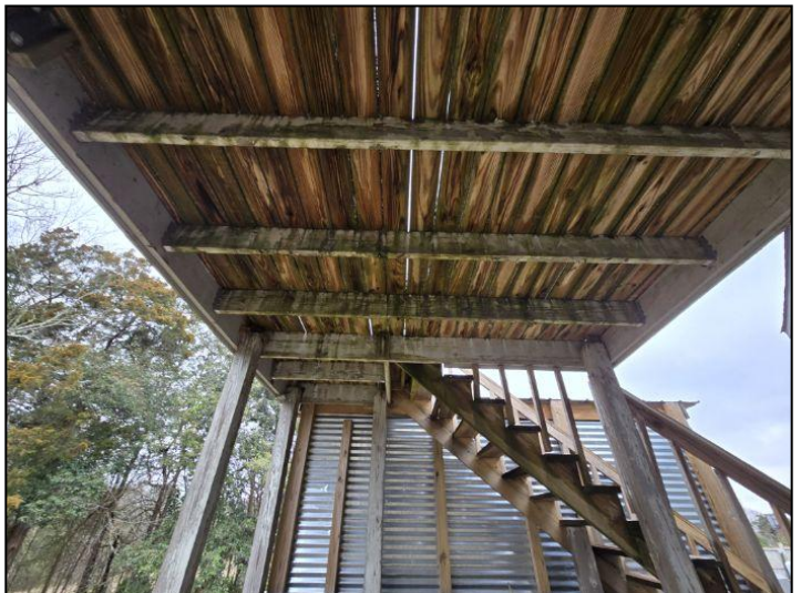
Possible mold growing under deck from severe water damage.
