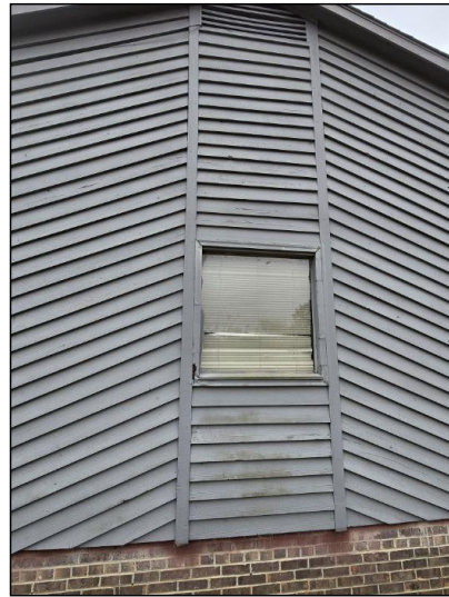
Some areas need priming and repainting.
