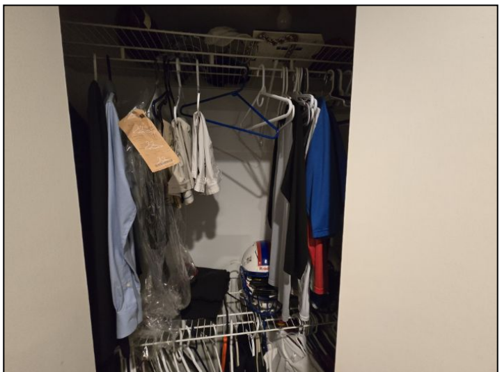
Left front bedroom closet light not working.
