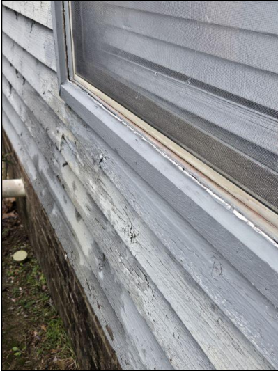
Some wood deterioration noted. Have repaired as necessary.
