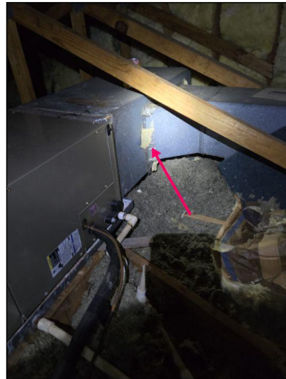
Wrapping is torn in areas.
